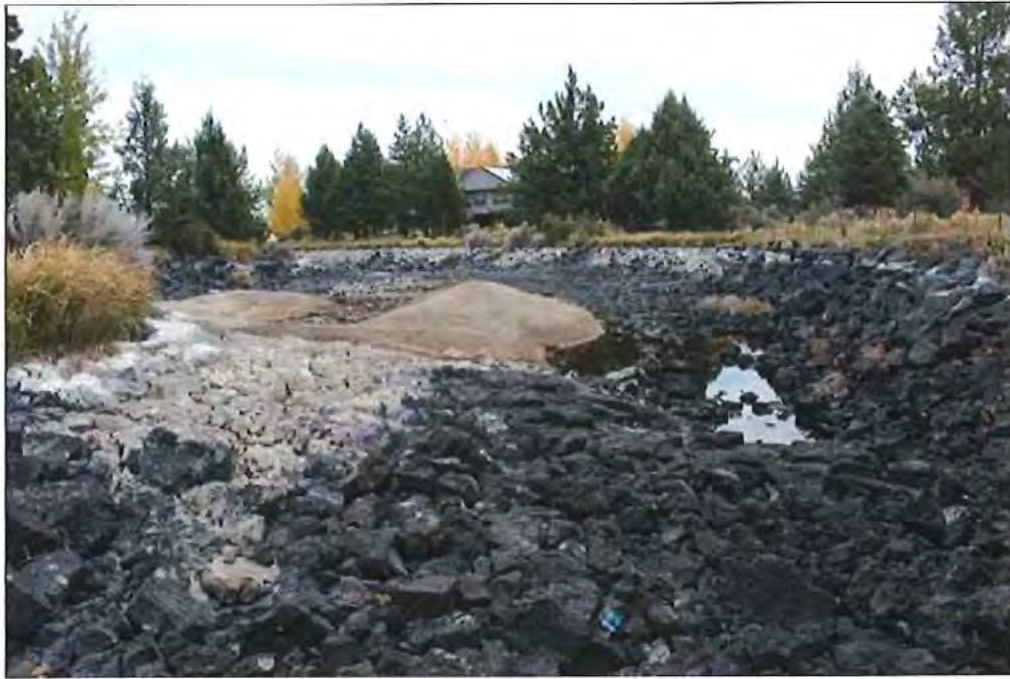
Photo 5 of 19: Segment 2. Canal is highly irregular in depth, width and side slopes, silt deposits, vegetated island in left foreground, looking north.
